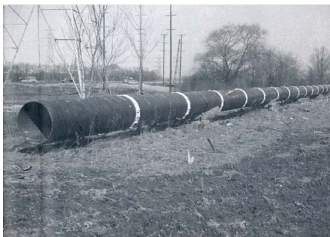
Circa. 1979, Model PE installed on steel pipe. Experience and today's application would target a steel casing spacer, or more PE's spaced at 6 ft. (1.83M).
